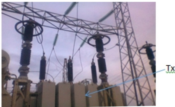
Figure 2: Damaged 132/33 kV 60MVA transformer (Tx)
